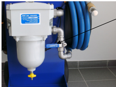
Shut off valve closed
